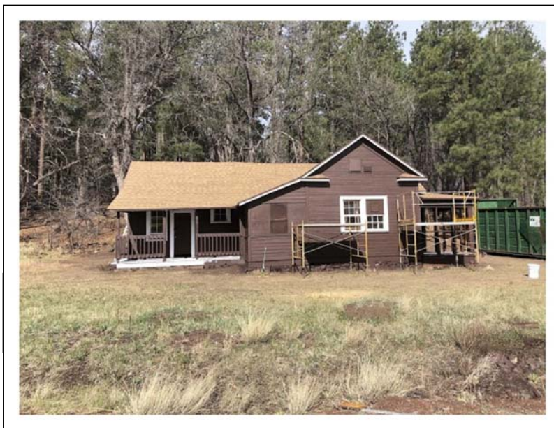
Mormon Lake Guard Station near completion of the 2018 project work, photo courtesy of HistoriCorps
