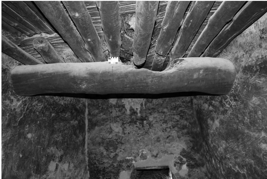
FIGURE 3. Original wooden ceiling at the Montezuma Castle cliff dwelling. Note evidence of burning on primary and secondary beams, right of scale card. Photo: M. Guebard.
